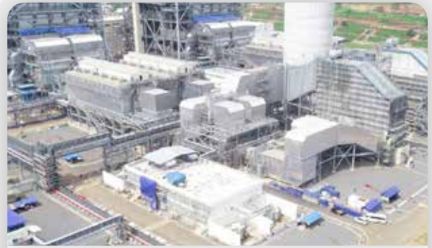
Sistem Penyaring Desulfurisasi Gas Buang dan Cerobong Flue Gas Desulfurization System and Stack
