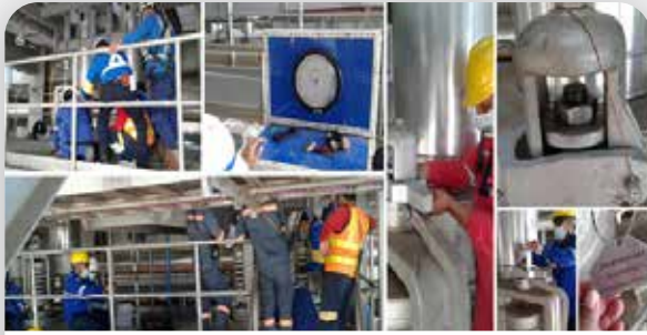
Inspeksi dan Pengujian Tingkat Pengaman Boiler U1 Inspection & testing of Pressure Safety Valve Boiler U1
