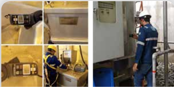
Inspeksi & pengujian Instalasi Listrik di area BTG Inspection & testing of Electrical Installation at BTG Area
