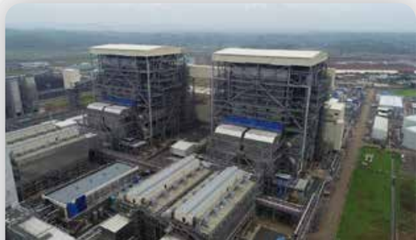
Ketel Uap & Penyaring Abu Terbang Unit #2 Boiler and Fabric Filter Unit #2
