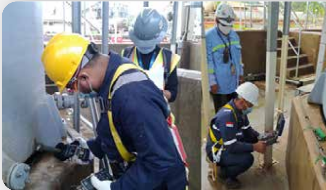
Inspeksi & pengujian Tangki Timbun di Area WWTP Inspection & testing of Storage Tank at WWTP Area
